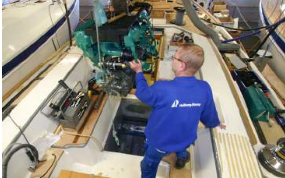
Engine and tanks come in through the normal opening of the boat after that the woodwork is done
