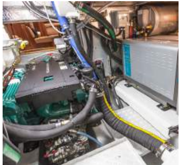
Large engine rooms. Easy access, easy maintenance. Everything is well sound insulated
