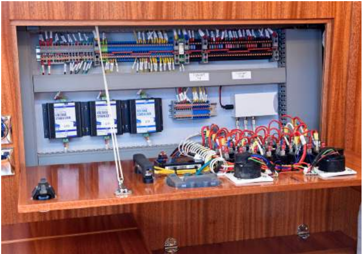
Easy fold out electric panel. All boats are delivered with individual wiring diagrams.
