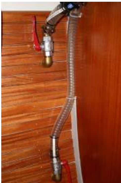
Easy access to well dimensioned ball valves for through-hull fittings
