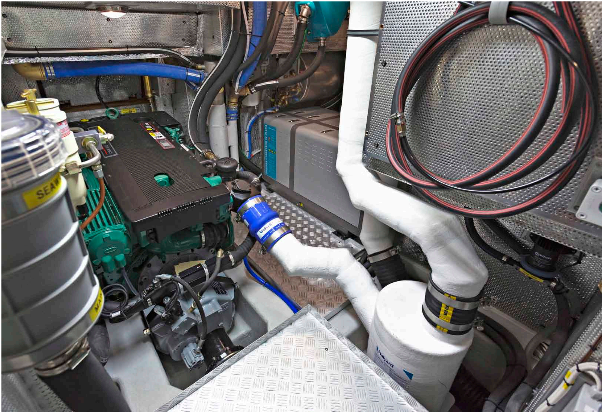
The big walk-in engine room allows for easy maintenance and good sound insulation
